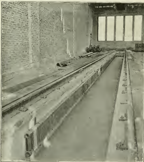
Typical Engine Pit.
